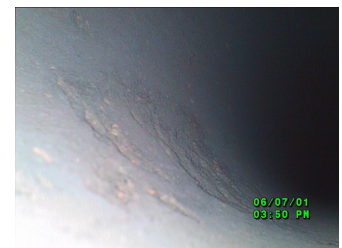
ID drum pitting found as a result of improper lay-up procedures on a coal fired boiler system taken out of service.
